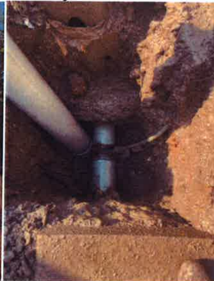
Old leaking saddle
