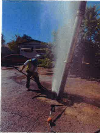
Leaking service line
