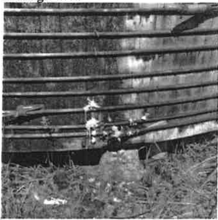
Photo #5: Tank Leakage Area
