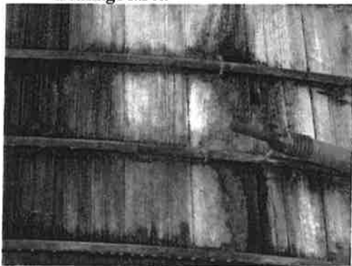
Photo #6: Tank Leakage Area
