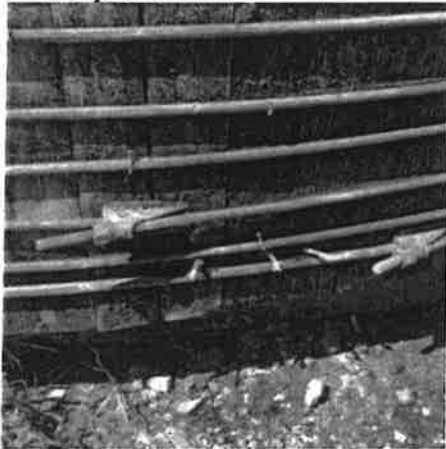
Photo #3: Tank Leakage Area
