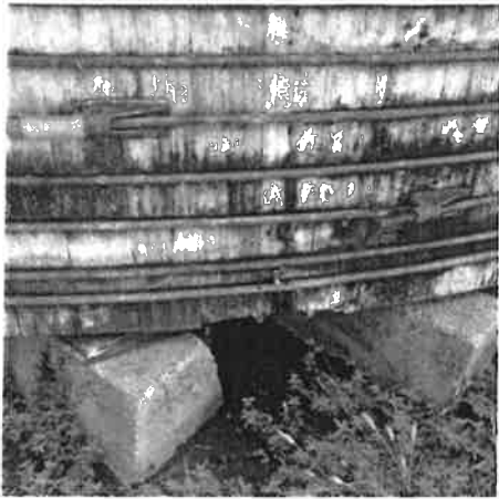
Photo #4: Tank Leakage Area
