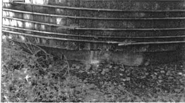
Photo #1: Tank Leakage Area
