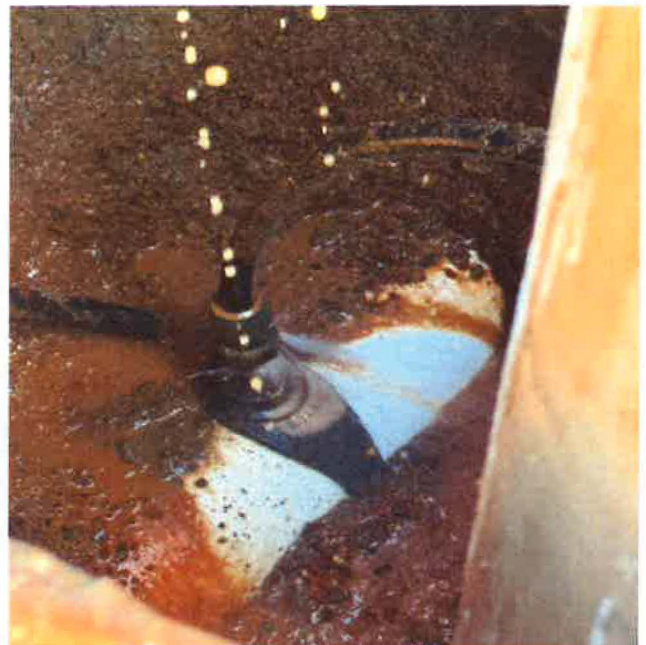
Corp stop leak on 4 th St
