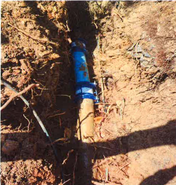
Main Leak on Island Circle x Blue Herron
