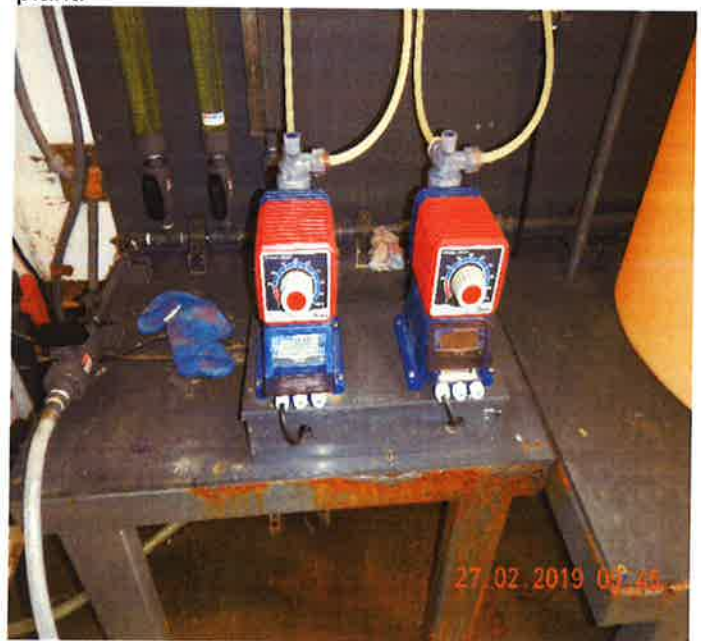
Photo No. 12: Chlorine injector pumps.
