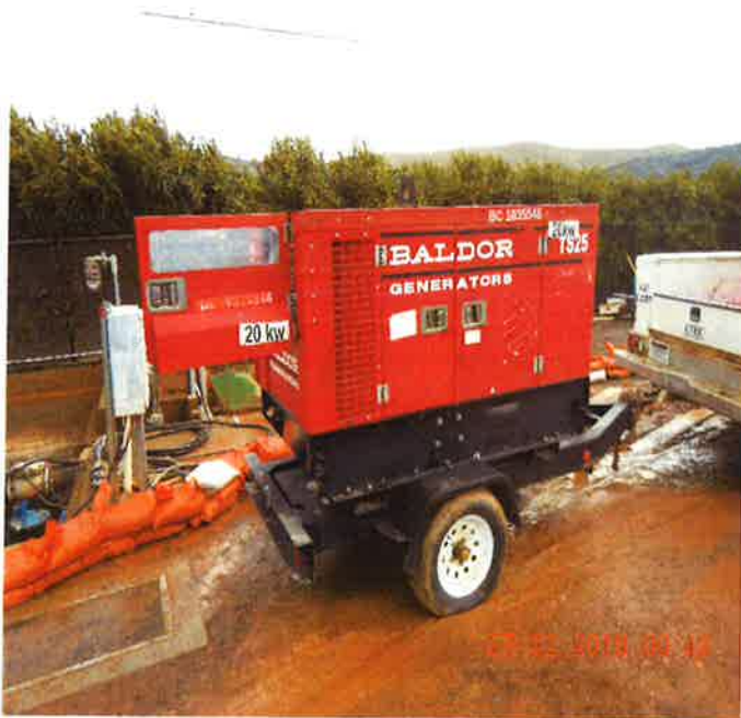
Photo No. 7: One of the portable generators used at the facility.
