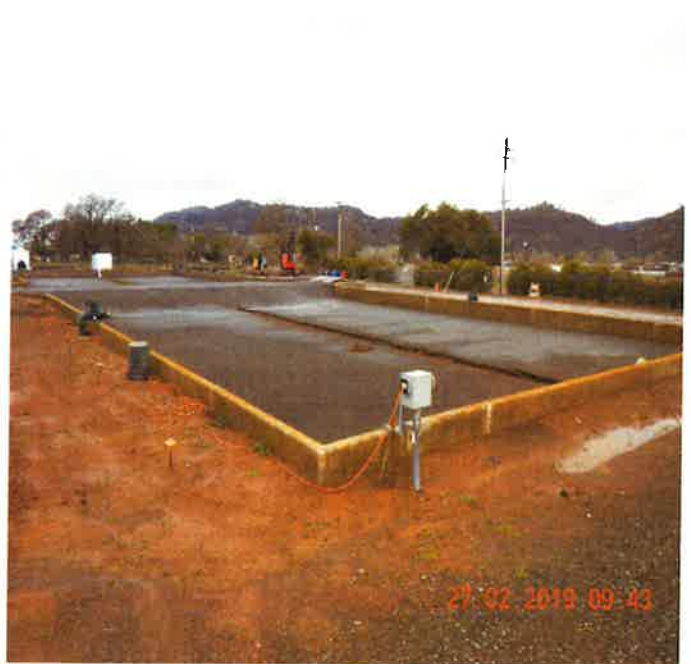
Photo No. 8: One of the four sludge drying beds at the facility.
