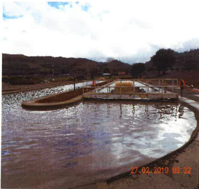
Photo No. 3: Aeration basin race track with two brush aerators.
