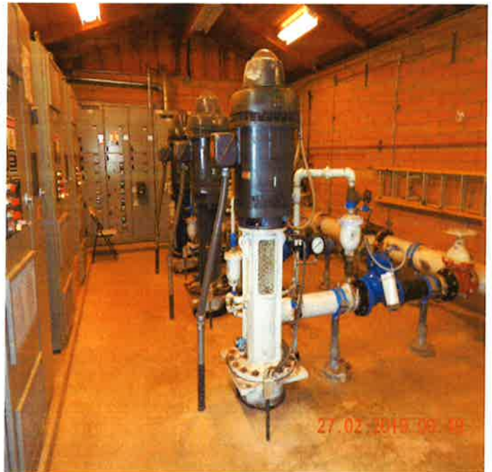
Photo No. 20: Effluent pumping station for transporting treated wastewater to the southeast geyser pipeline for disposal.
