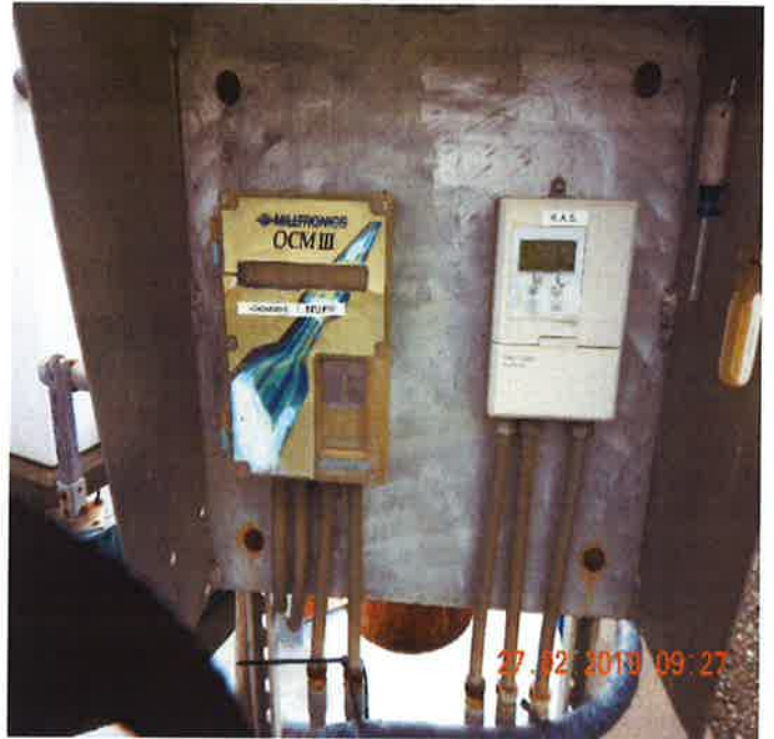
Photo No. 2: Influent flow meter.
