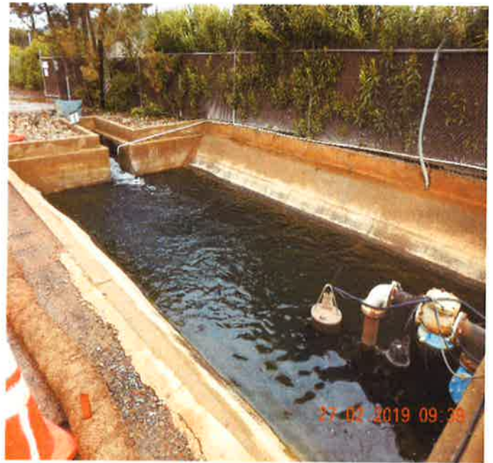
Photo No. 6: Clarifier effluent pump station.
