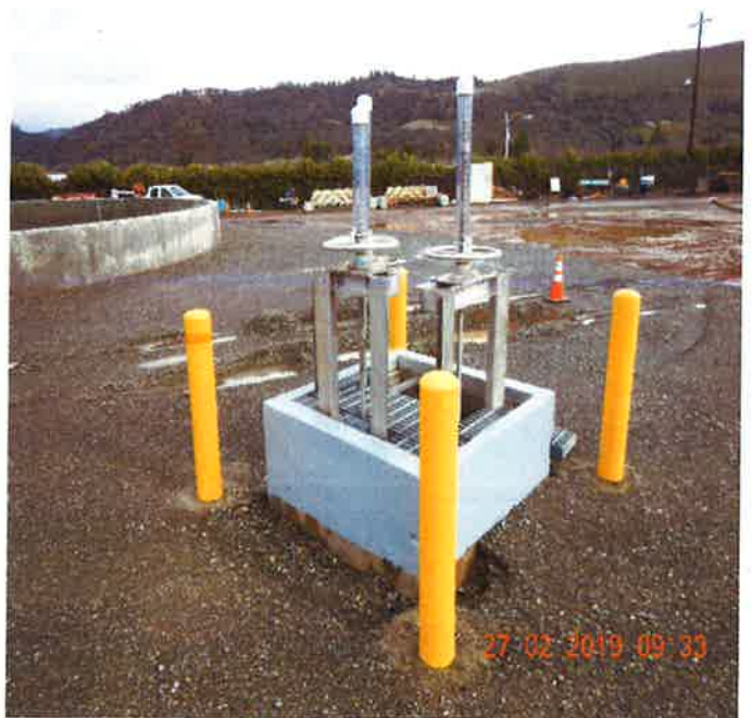
Photo No. 4: Flow splitter box at the treatment plant.
