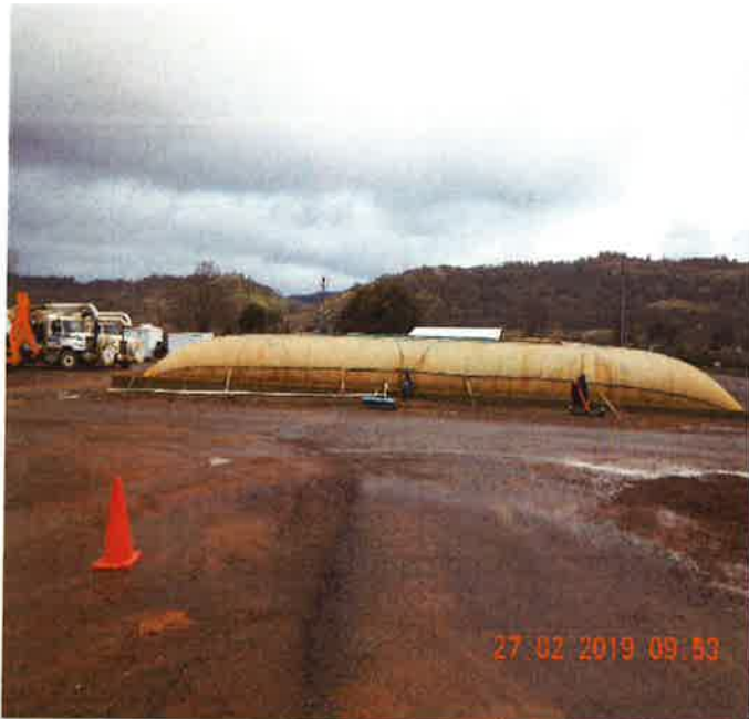
Photo No. 9: Looking west at Geotube bags located within the sludge drying beds.
