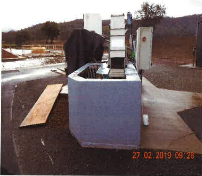
Photo No. 1: Headworks and bar screen.
